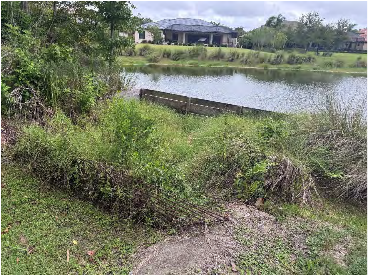
Figure 8 - Pond 40 Outfall Overgrowth
