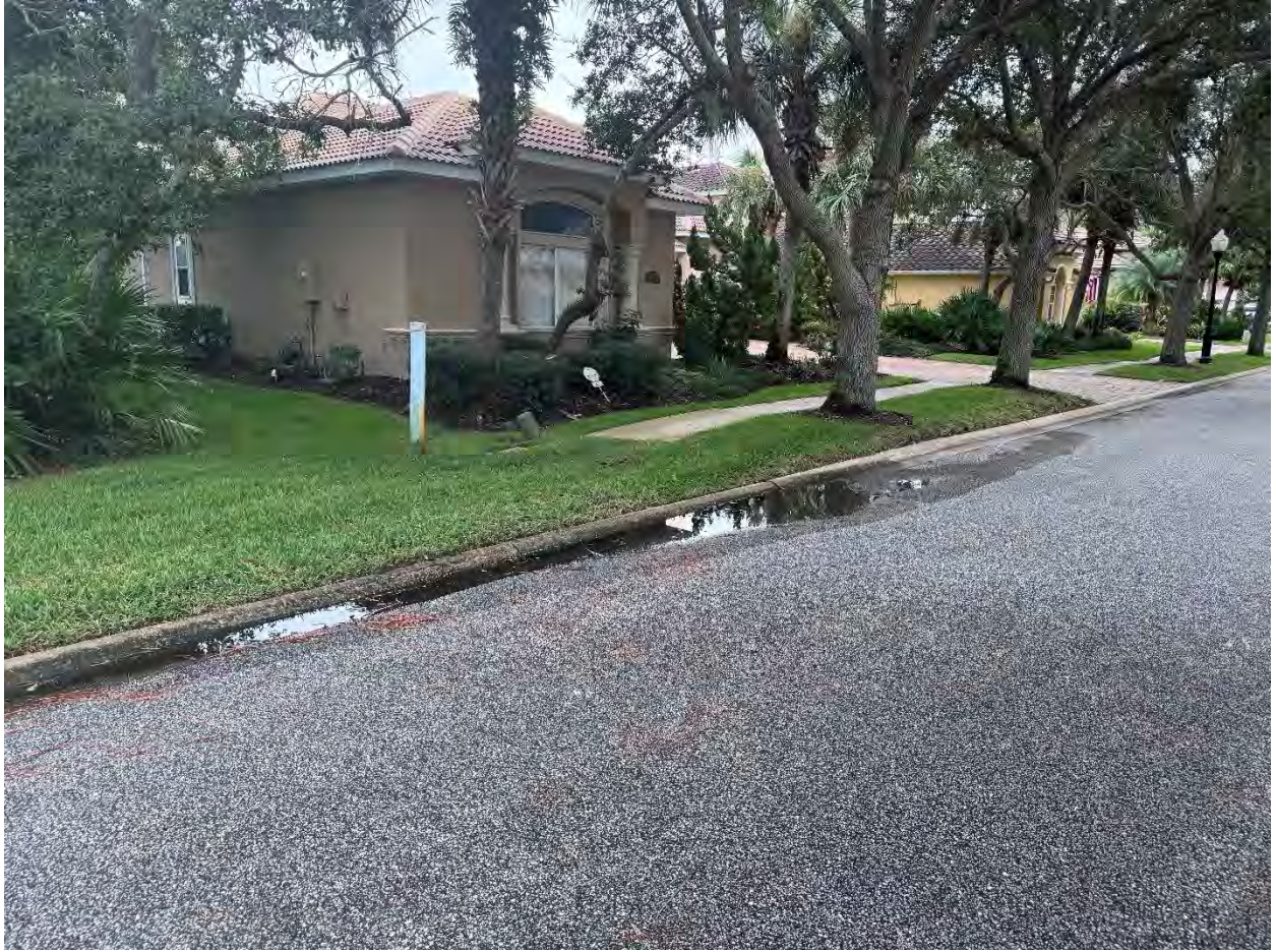
Figure 17 - Curb and Gutter Holding Water
