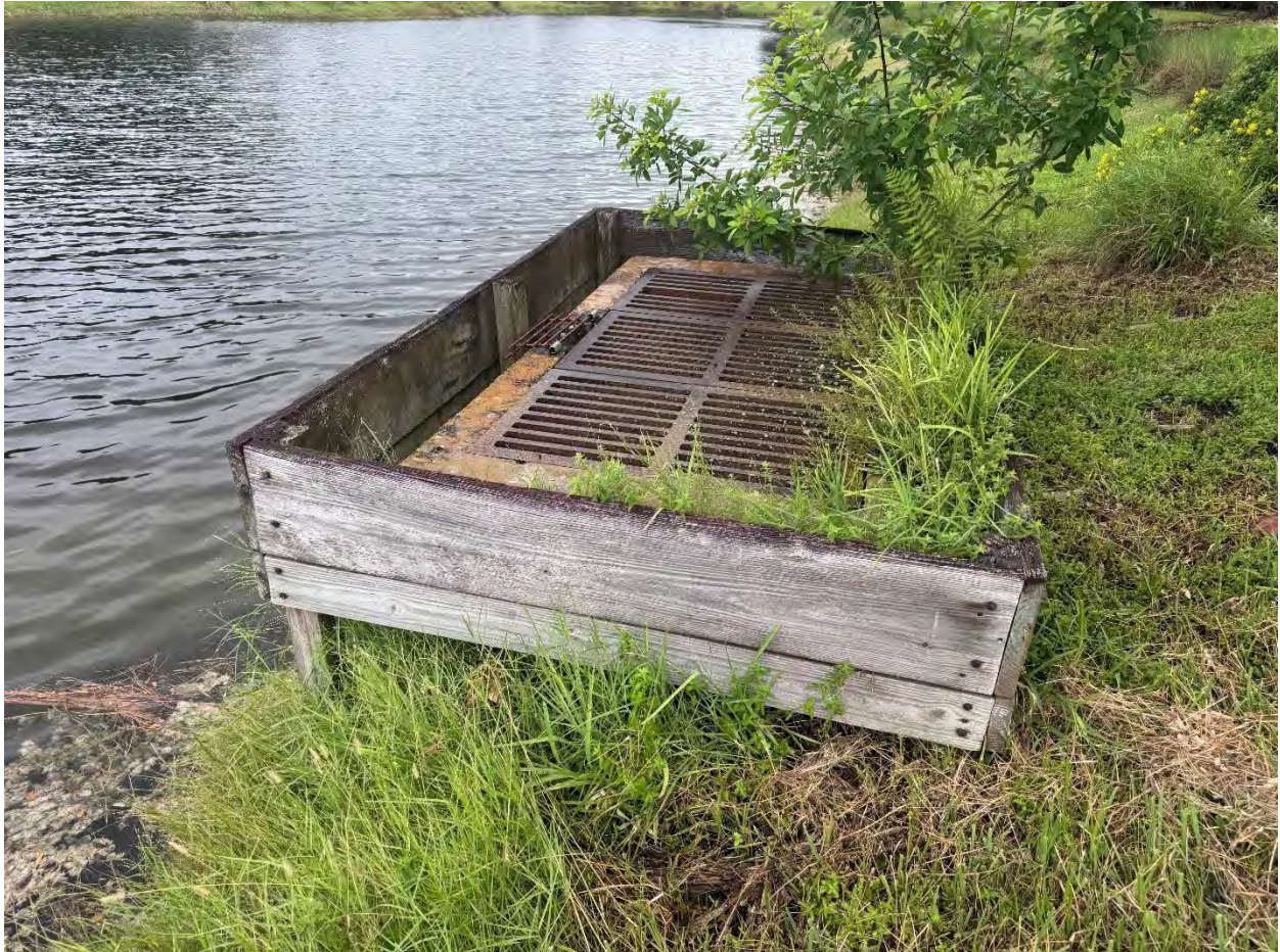
Figure 9 - Pond 28 Control Structure Overgrowth
