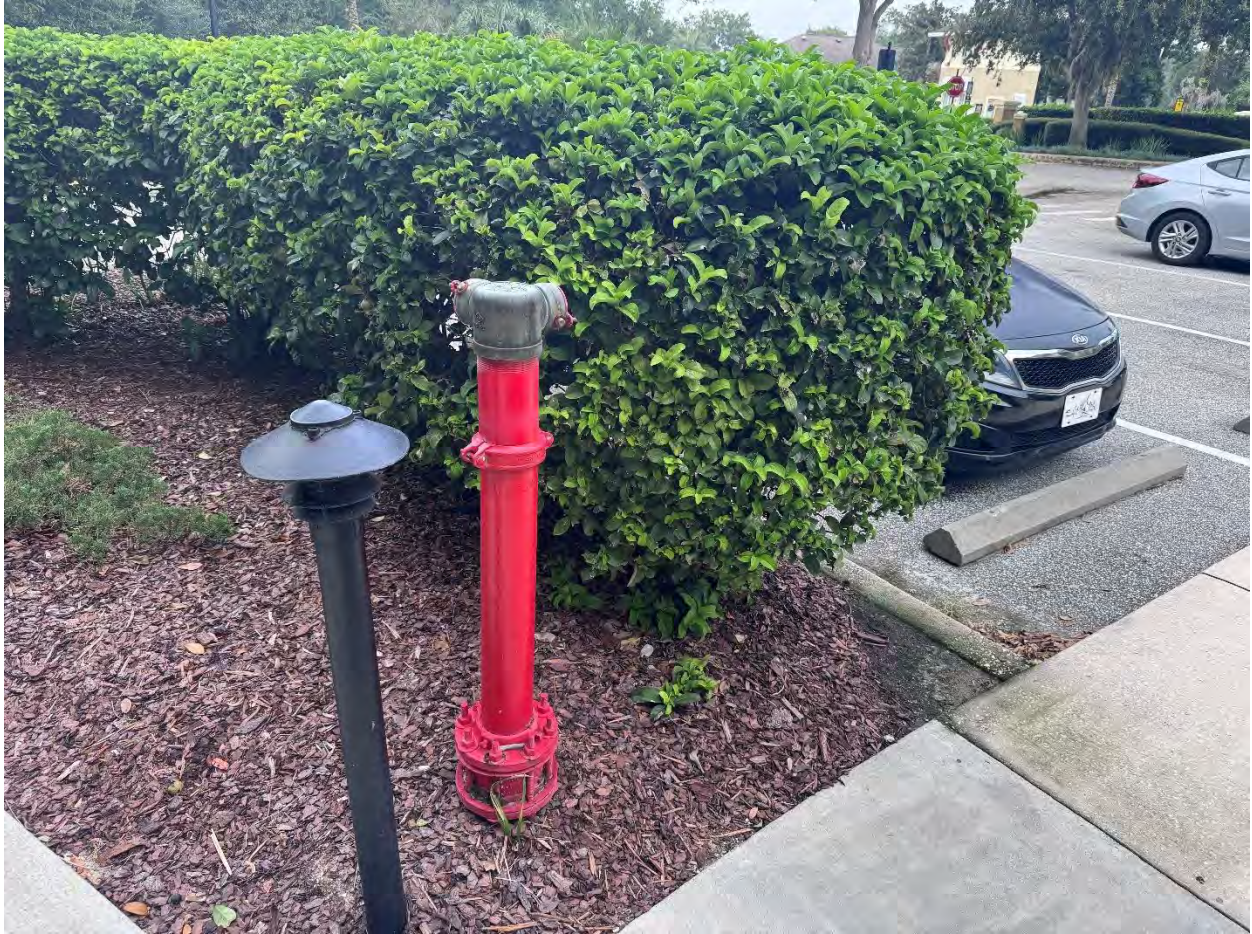
Figure 1 - Creekside Amenity Center FDC
