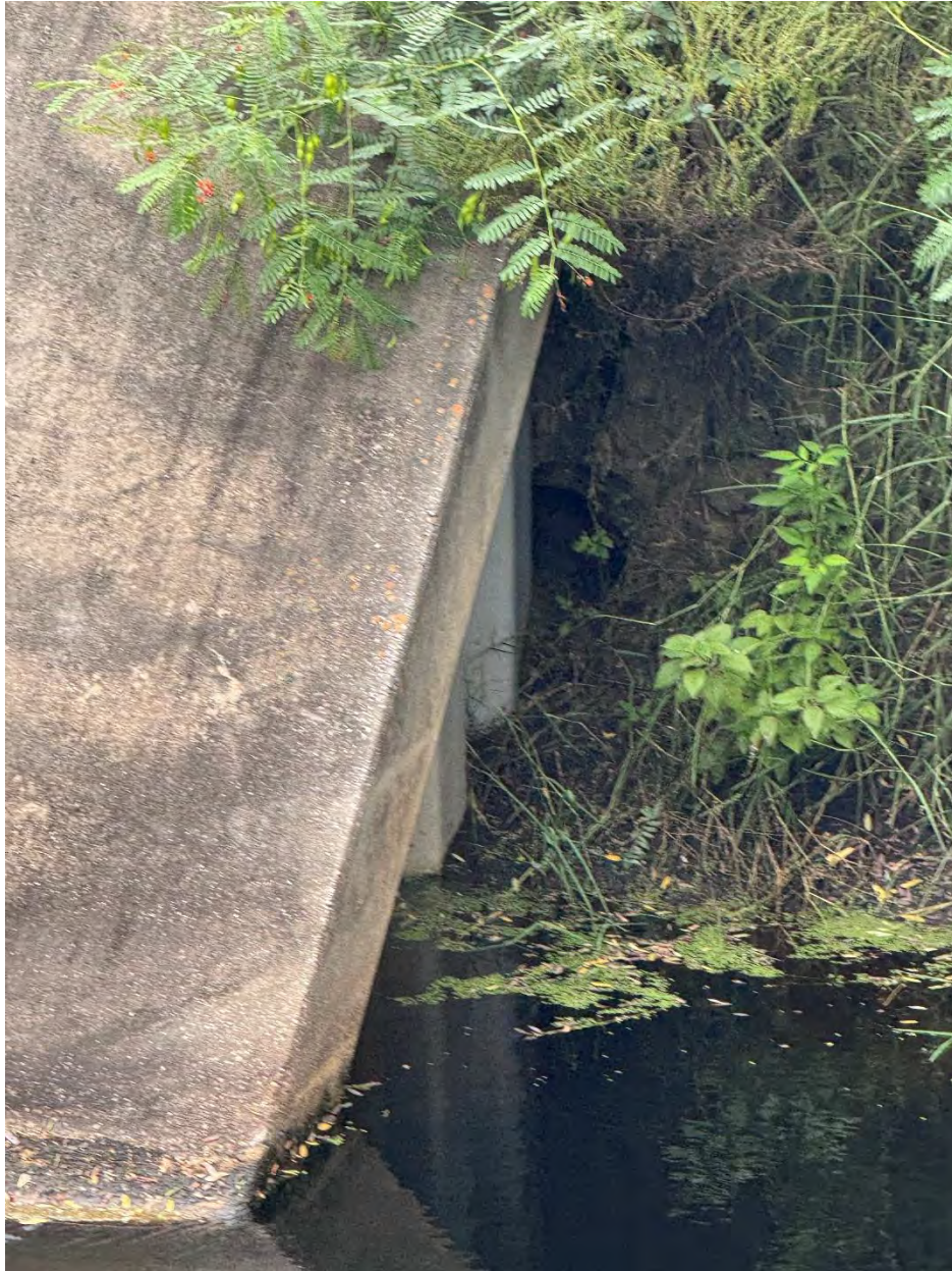
Figure 7 - Sheet Pile Wall Scour
