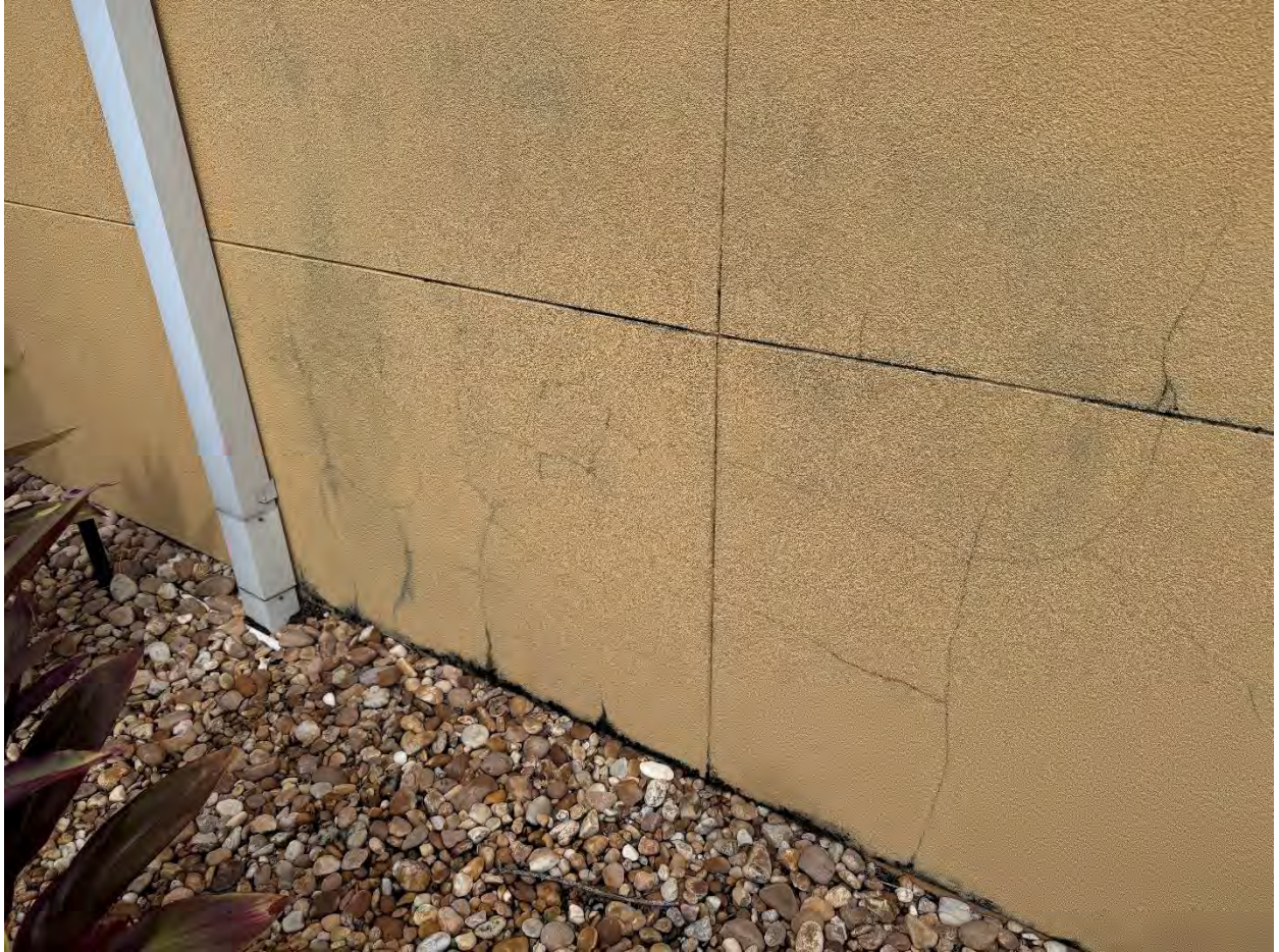
Figure 4 - Amenity Center Wall Mildew and Wicking
