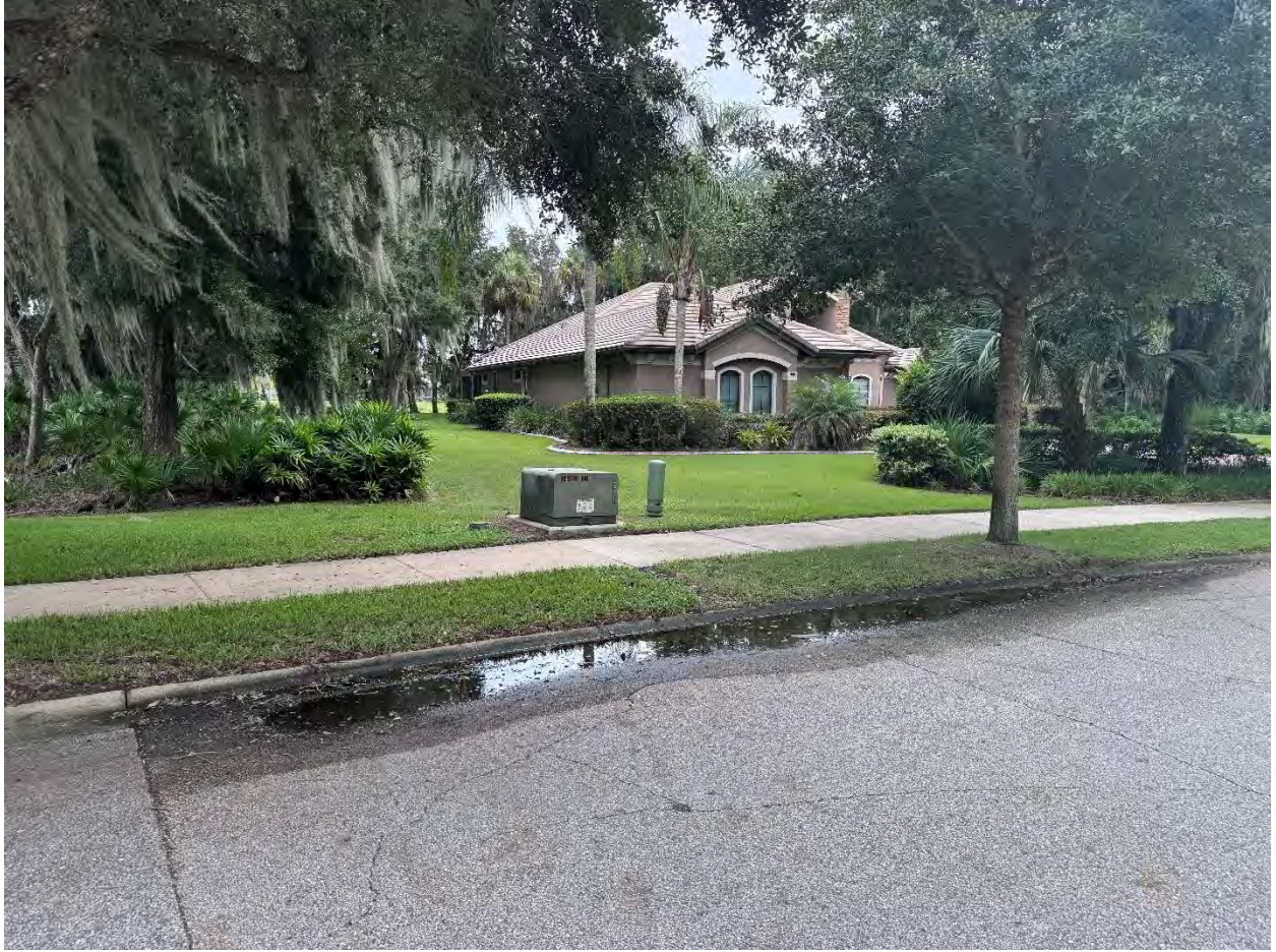
Figure 16 - Curb and Gutter Holding Water
