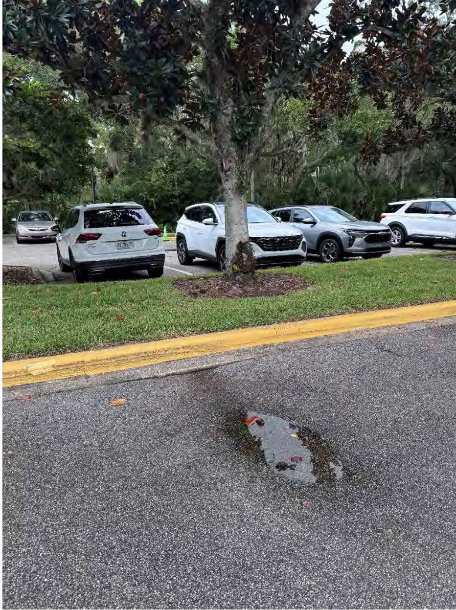
Figure 5 - Depression in Parking Lot
