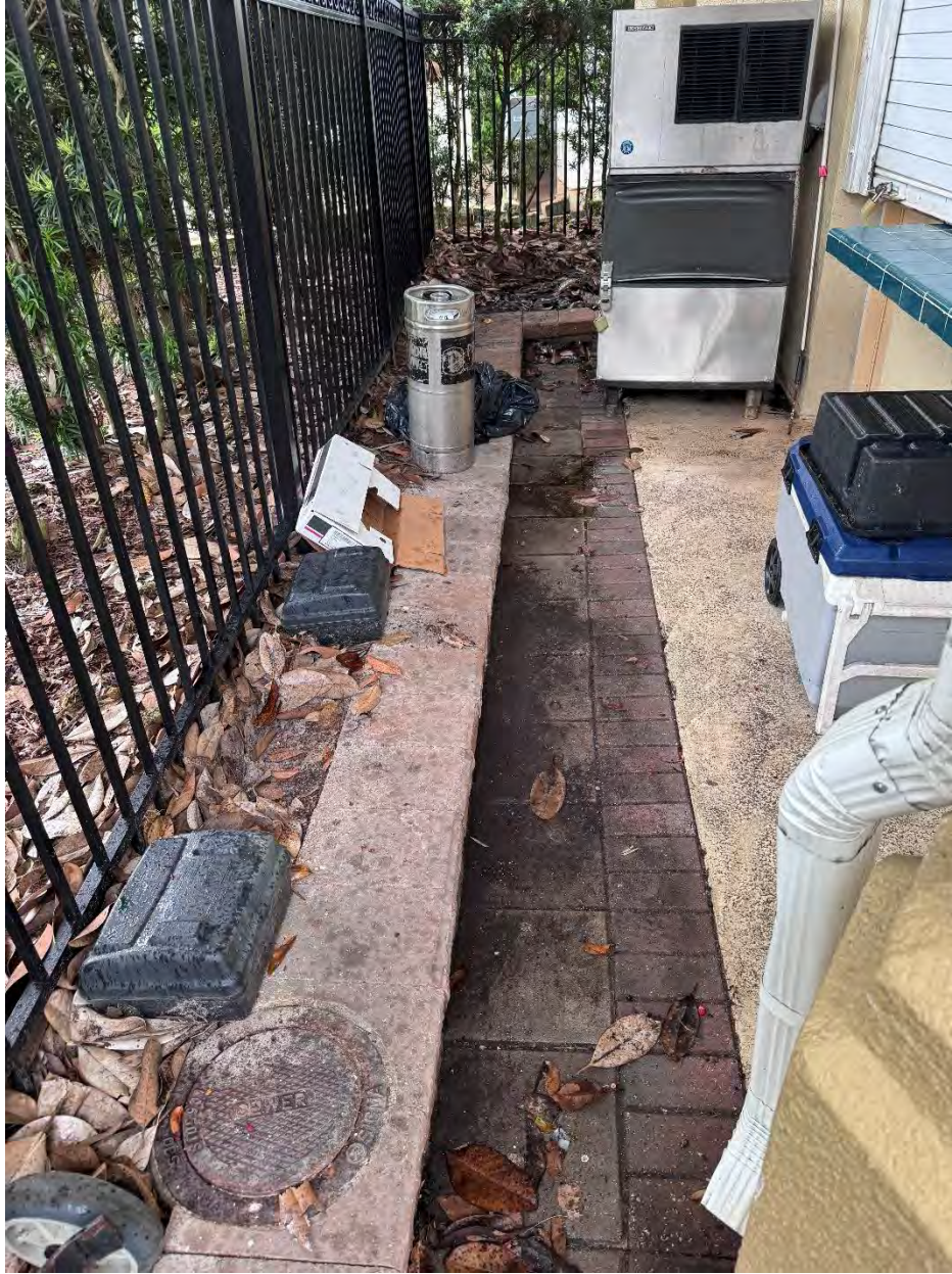
Figure 2 - Tiki Bar Flooding
