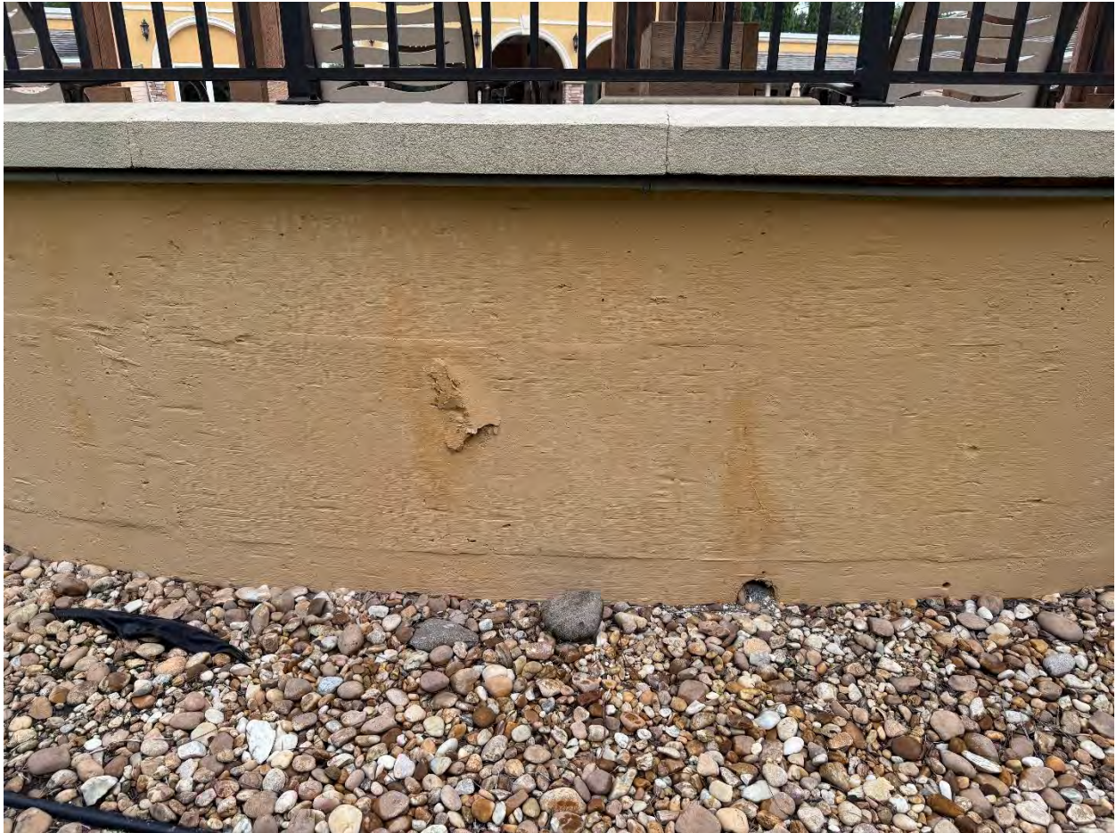
Figure 3 - Retaining Wall Spalling
