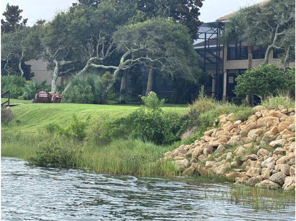
Figure 10 - Pond 28 Outfall Overgrowth
